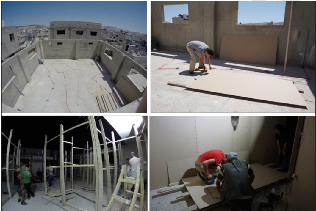
Images showing the gradual process of building up the roof scale, while responding to the contracting “working space”: (TL) Jami’yeh Roof with taped layout, Top Right: Commencing of the building process, (BL) most of the wall frames erected, (BR) final building stages, Baqa’a camp, Jordan 2015. © Samar Maqusi
